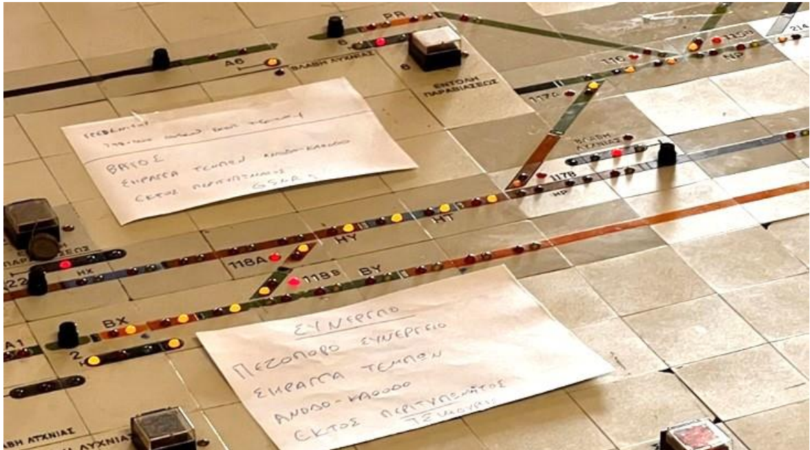
Figure 48. Detail of the Larissa Control Panel with a route set to cross a switch in a bypass position.
