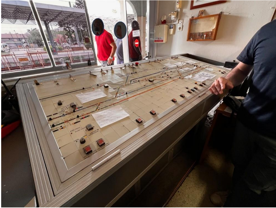
Figure 37. The control panel at Larissa Station
